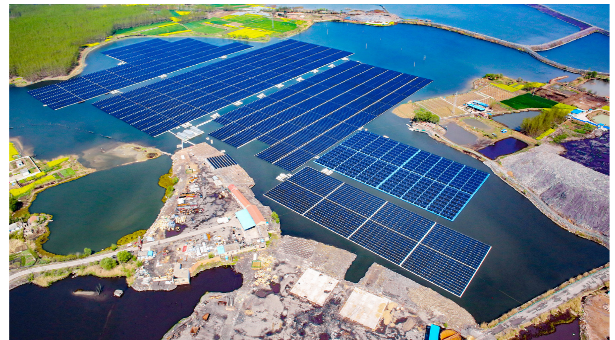
Huainan Solar Farm, with an approved grid-connected capacity of 20MW 淮南電站，核准併網容量20MW
