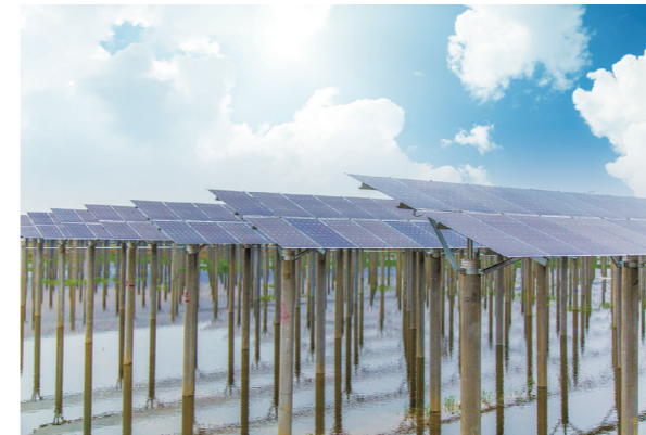
Shouxian Fishery-PV Complementary Solar Farm 壽縣漁光互補電站
